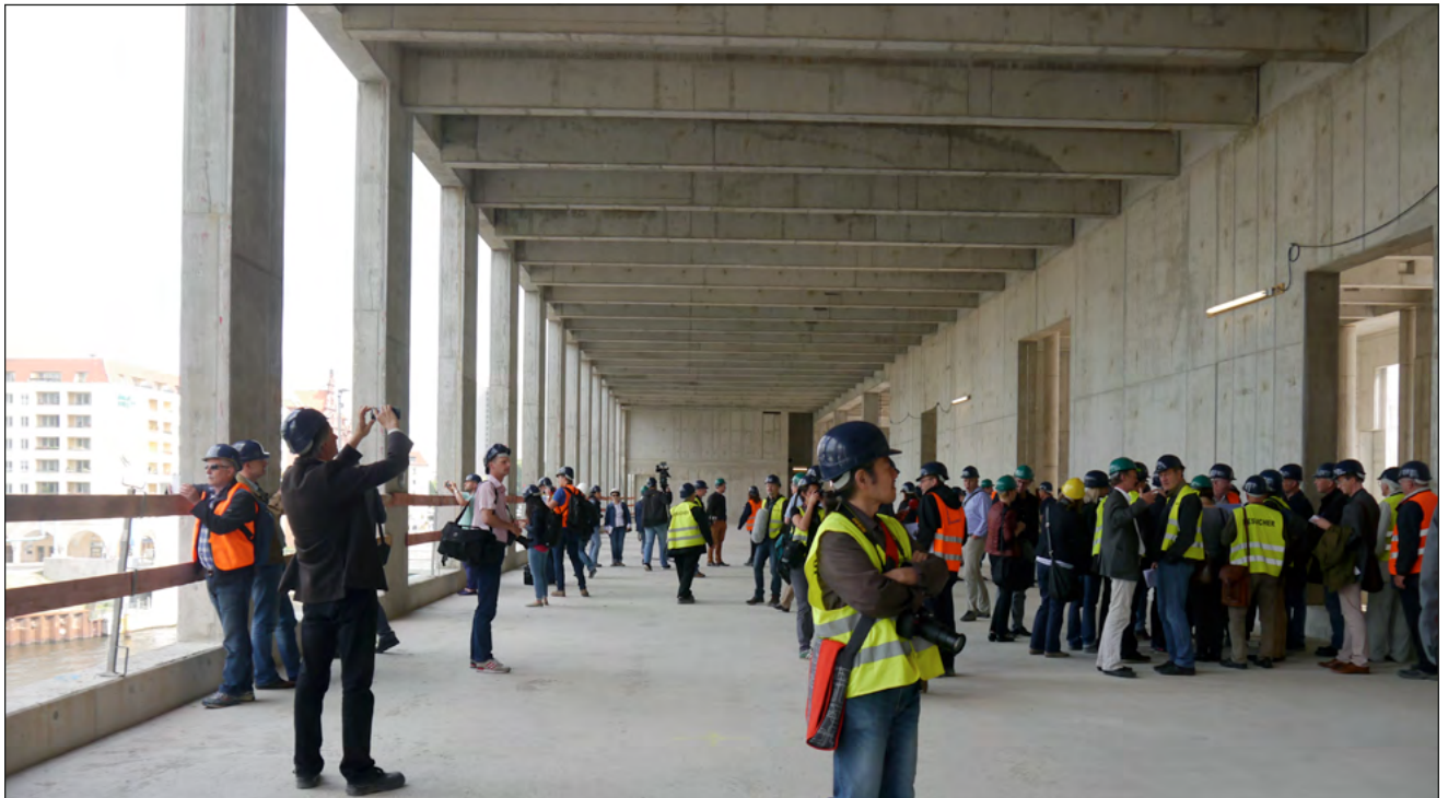
Around 200 representatives of the media were present at the first official tour of the Humboldt Forum construction site, one week before the official topping-out ceremony. (Photo: Claudia Lamas Cornejo | BWG 2015)
